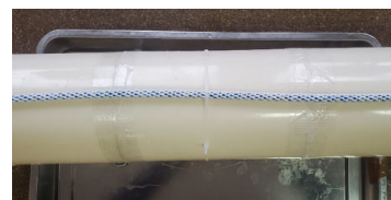
The sense cable is fastened at the 6 o'clock position beneath the pipe, positioned centrally under the pipe. (The photo is captured from beneath the pipe)
