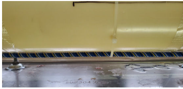
The cable is neatly and securely attached on the pipe base.
