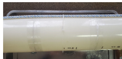
The sense cable is fastened on the side of the pipe base.
