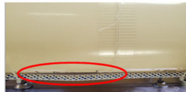
Poor contact between the cable and the pipe base.
